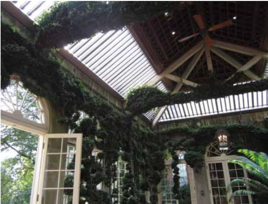
The Orangery now boasts better catering and restroom facilities, as well as a beautifully renovated roof.
